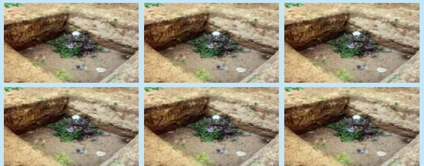
Six more pits were added in M.Sc. and B.Sc. Hostel areas to contribute towards improving the ranking of the city in the "Swachhta Sarvekshan-2022".
