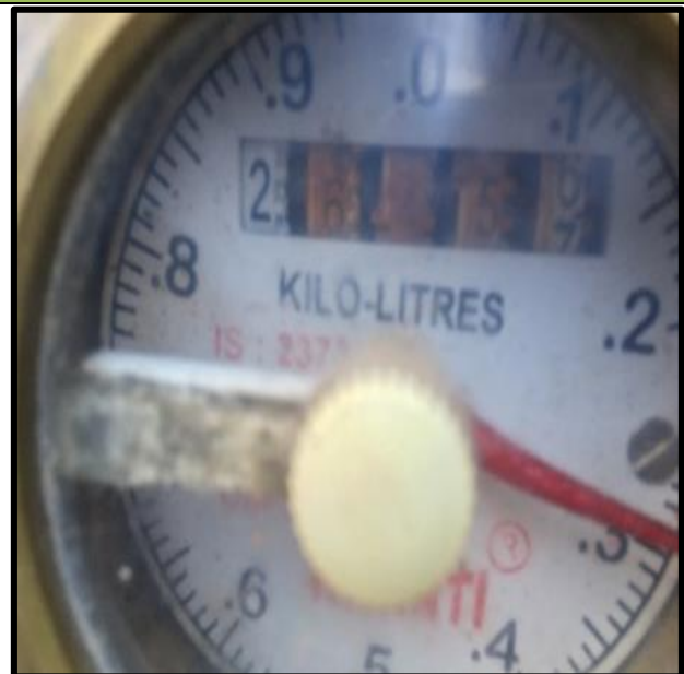
Water Meter of M.Sc. Block
