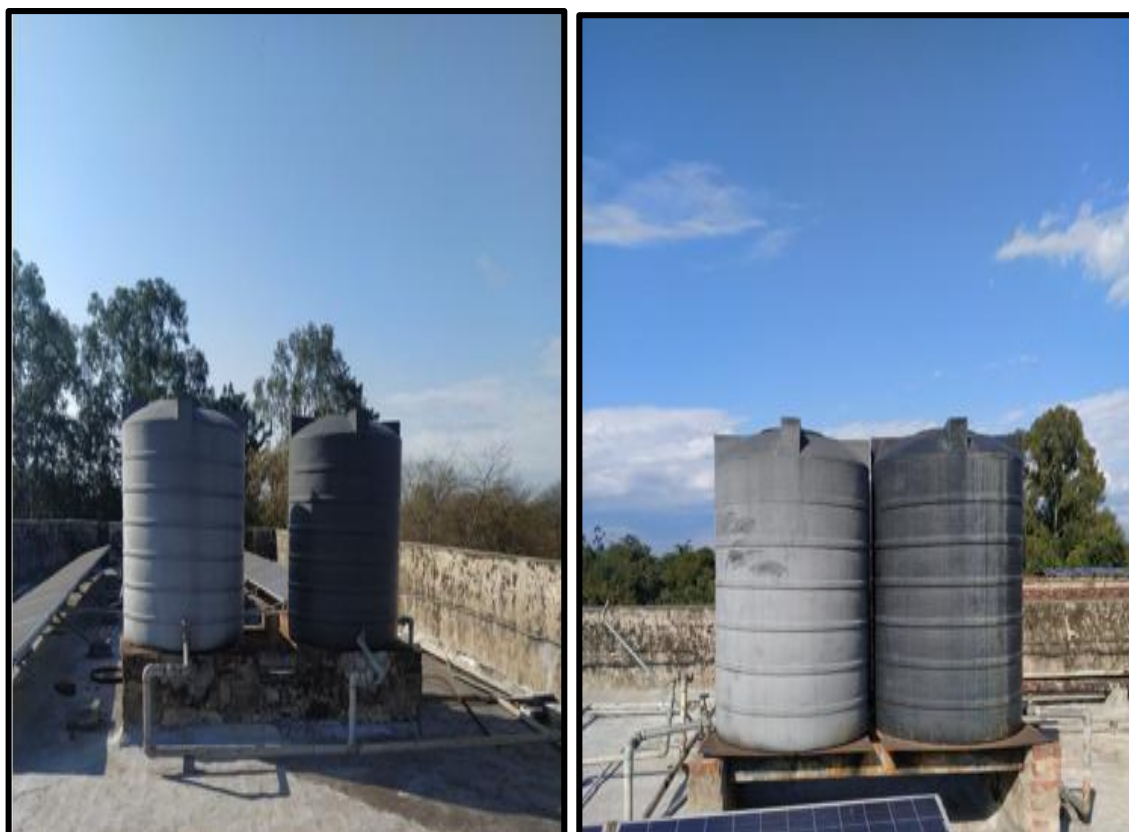
Water Storage Tanks
