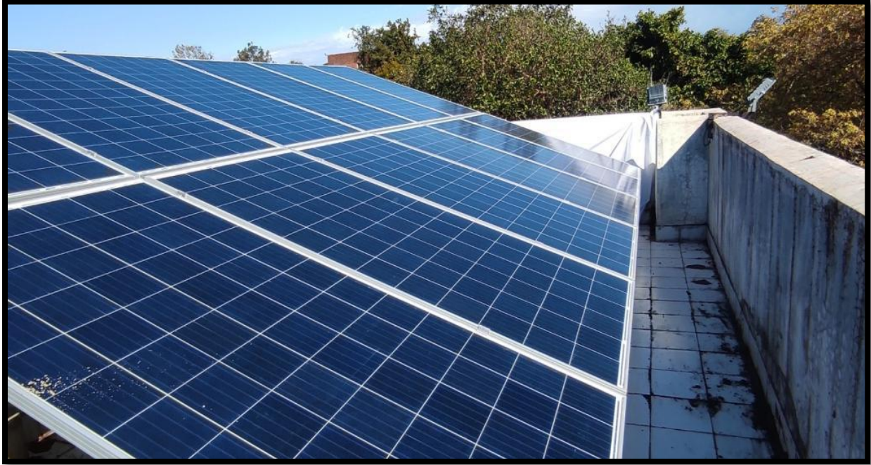
Solar Panel on the Main Academic Building
