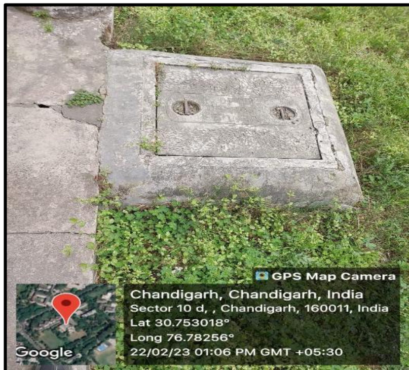
Collection pits having connecting from Rooftop to ground water through R.C.C. Pipes
