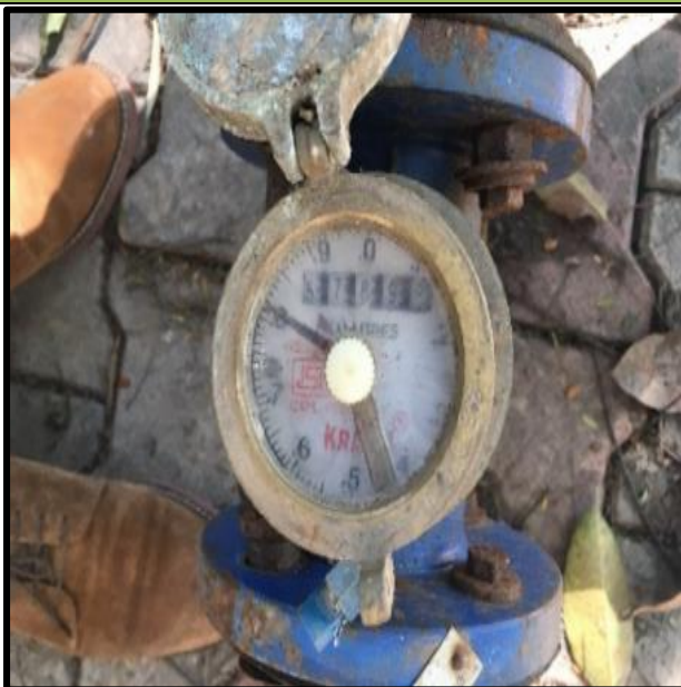
Water Supply meter near Academic Block
