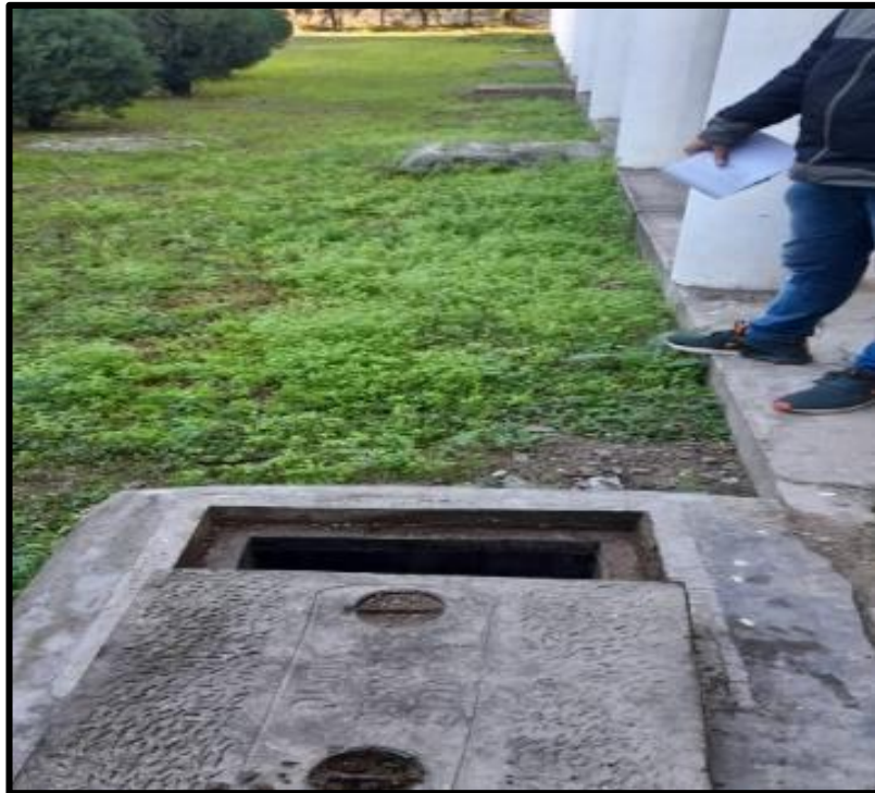
Collection pits having connecting from Rooftop to ground water through R.C.C. Pipes
