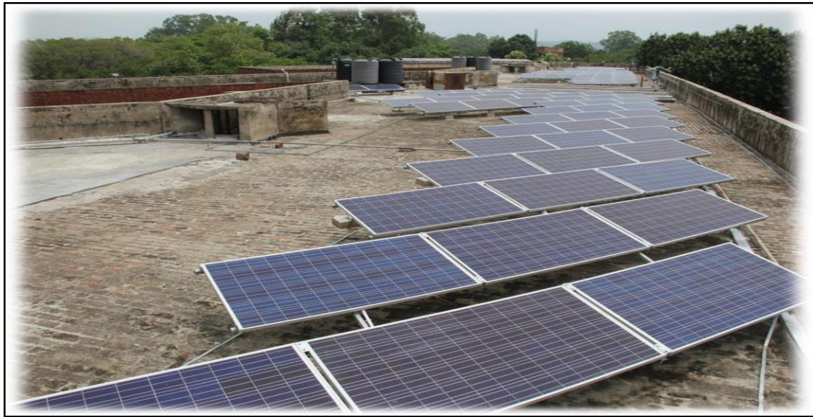
Solar Panels on P.G. Hostel Building (30kWp)
