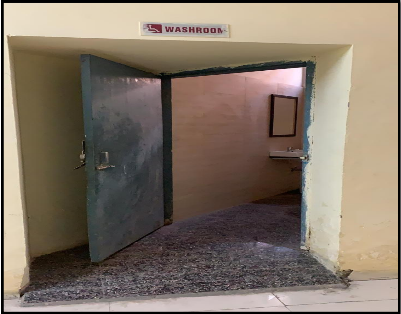
Disabled Friendly Washroom
