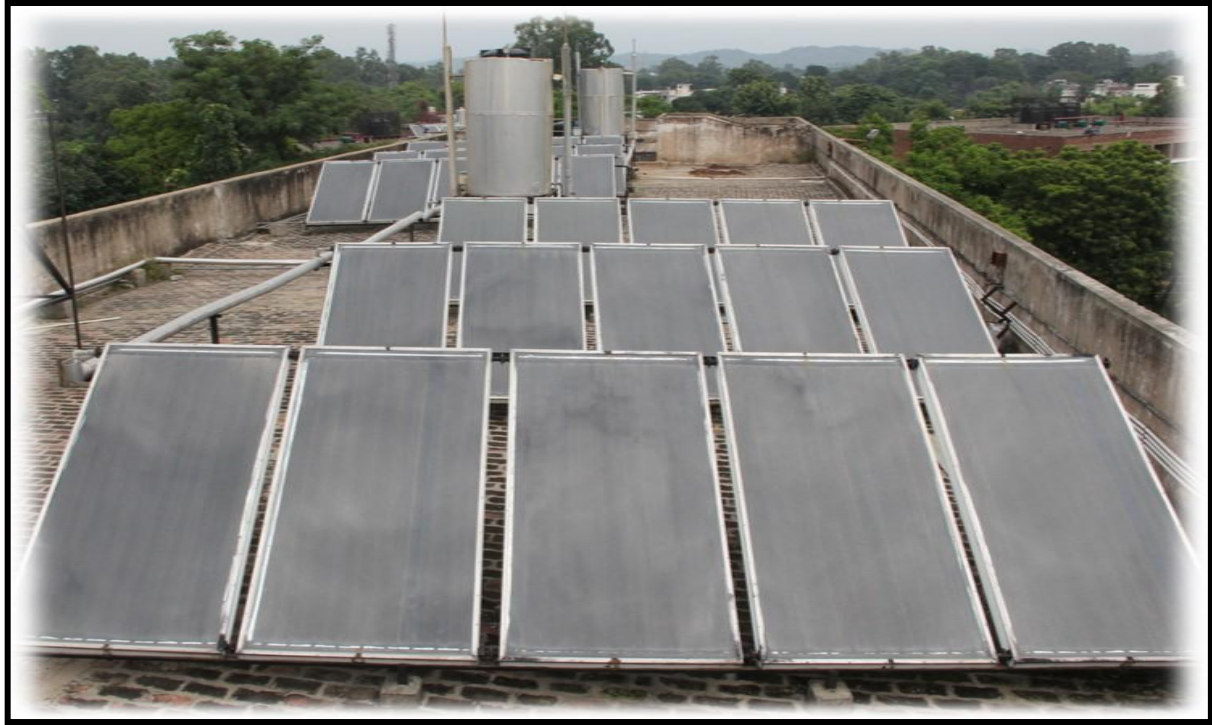
Solar Panels on U.G. Hostel Building (2 x 25kWp)
