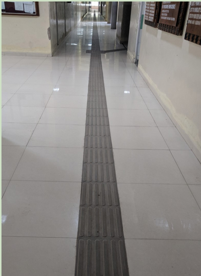
Vitrified tactile tiles on the ground floor to make college disabled friendly
